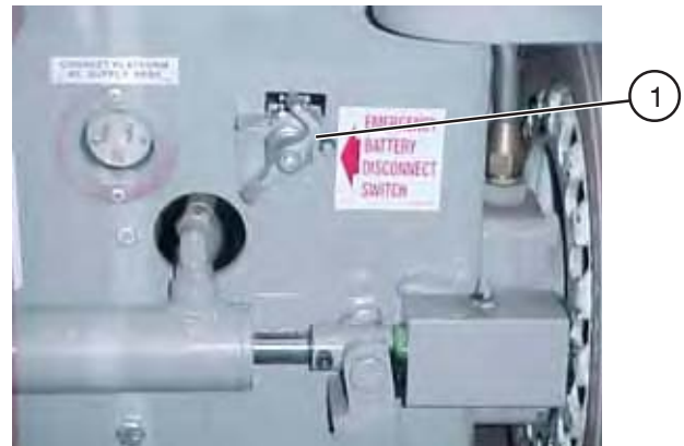
Figure 2-2. Emergency Battery Disconnect Switch
